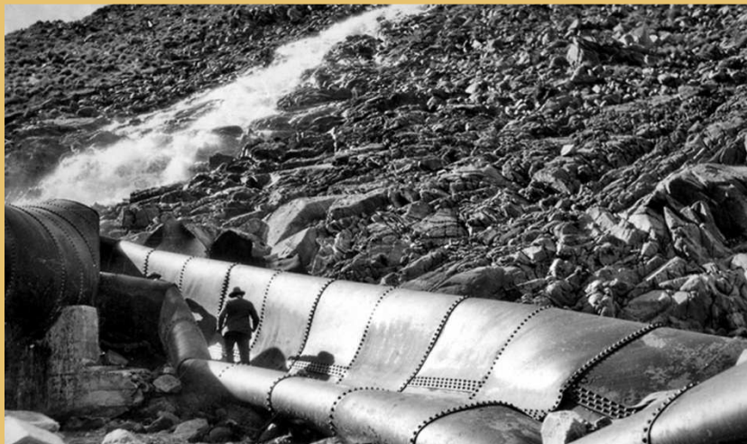
Aqueduct Dynamited south of the Alabama Gate in No Name Canyon – 1924
